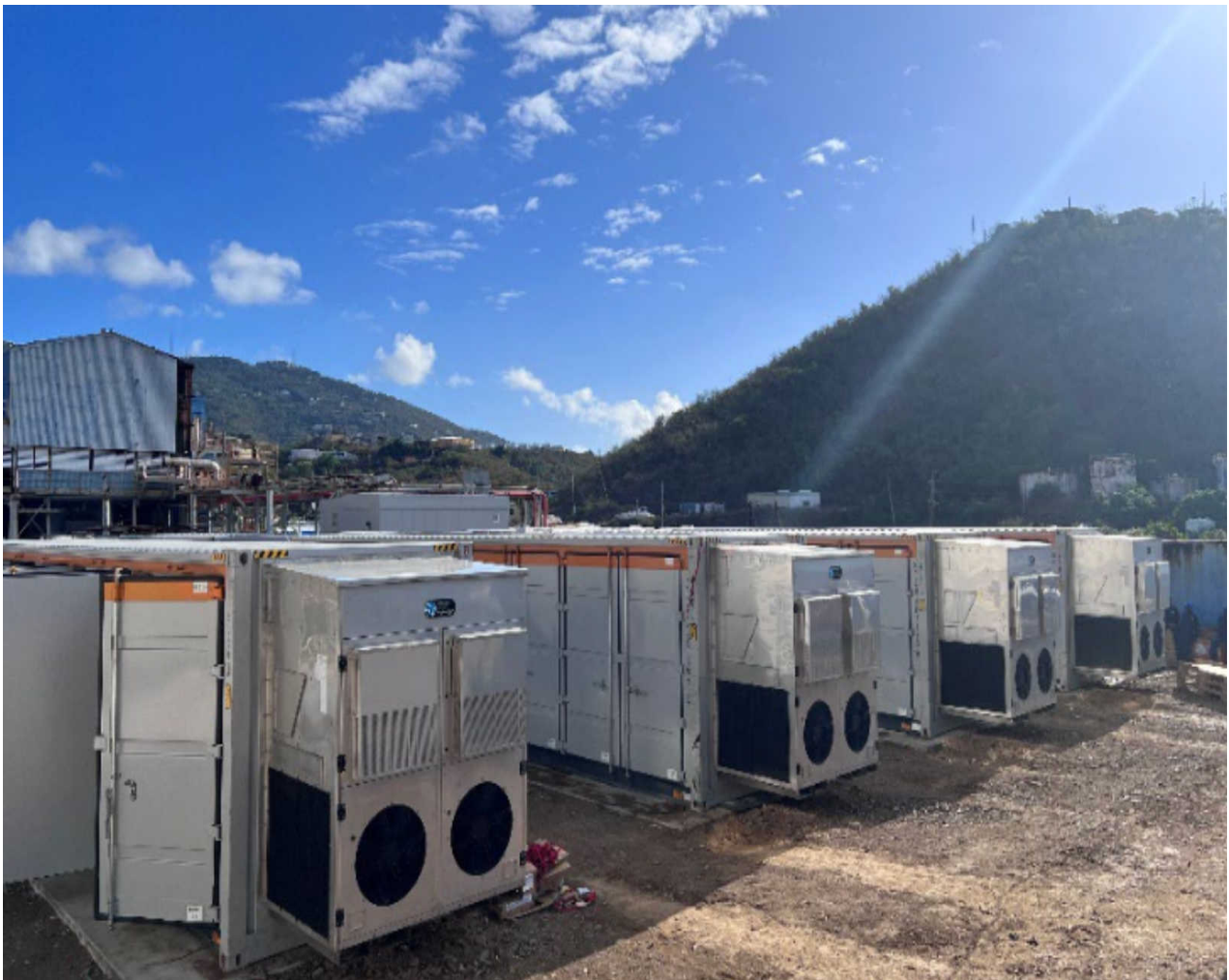
Several Battery Energy Storage Systems at the Randolph Harley Power Plant in St. Thomas. By. WAPA
