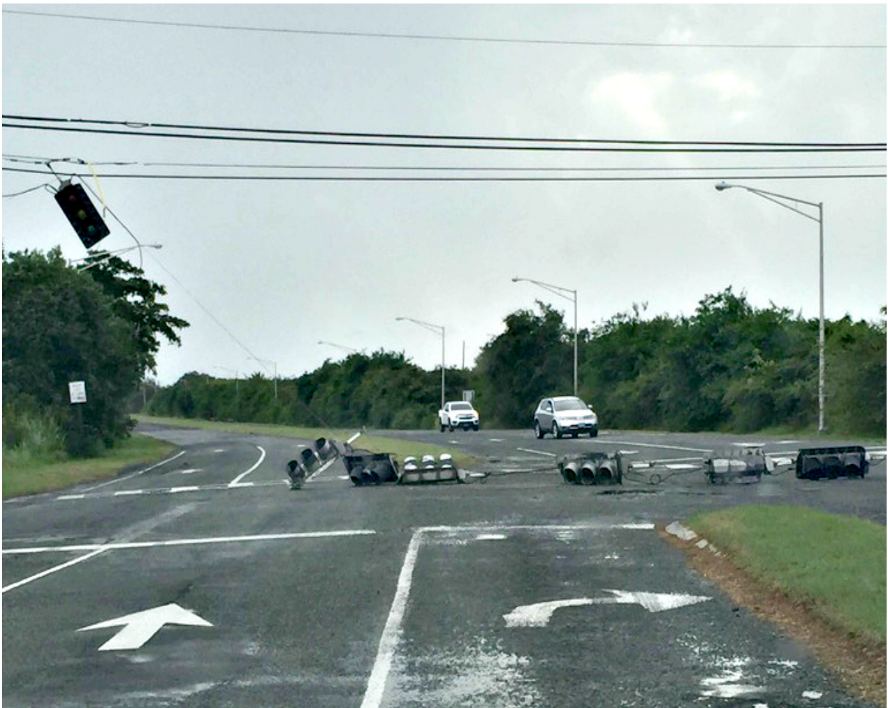
Destroyed traffic lights on St. Croix following Hurricane Maria in 2017 By. ERNICE GILBERT/VI CONSORTIUM
