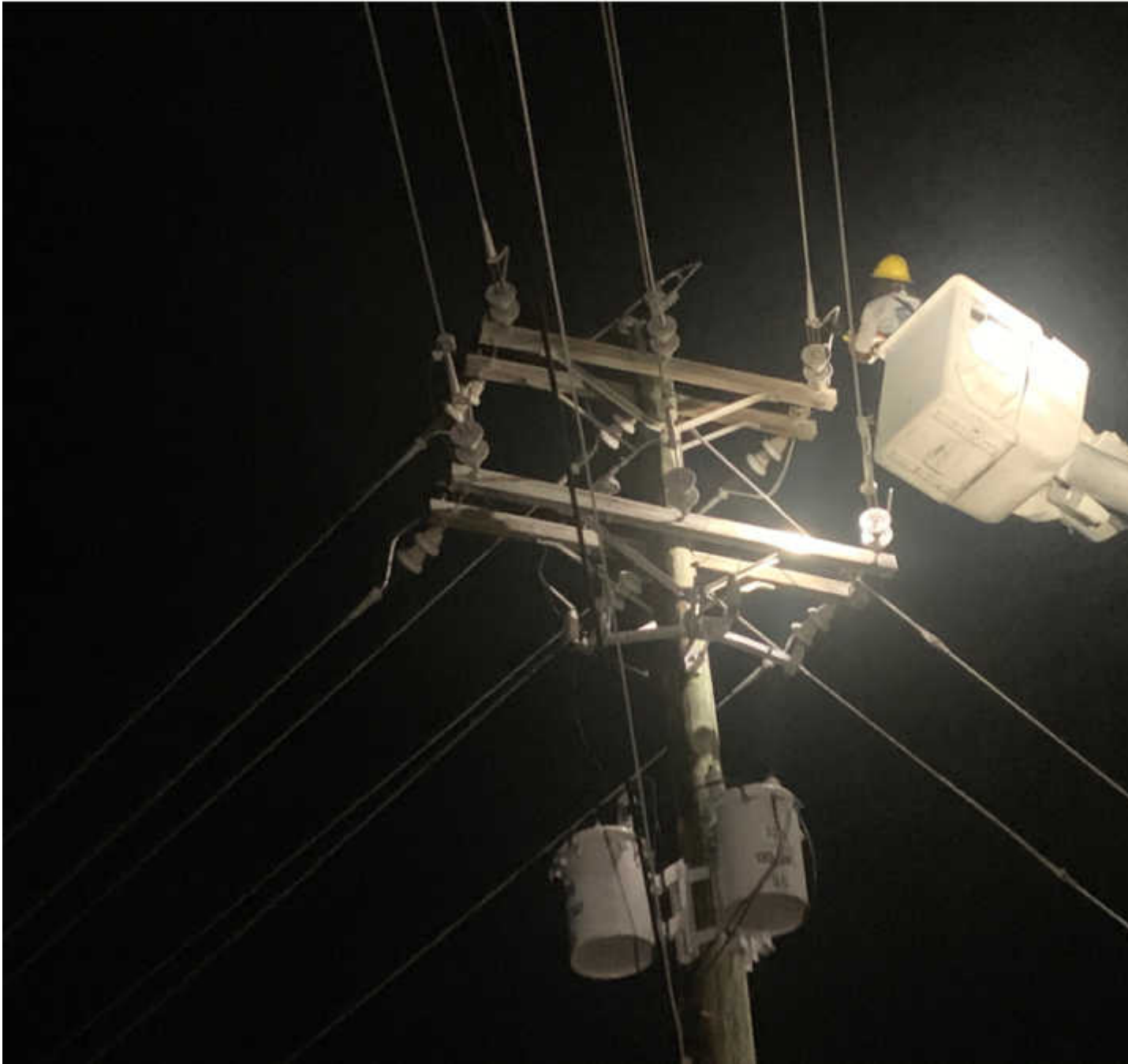
WAPA Line Supervisor Malvern Williams works on a pole in Subbase St. Thomas following a fire which destroyed circuits associated with two electrical feeders. The pole fire was the cause of a districtwide outage on Sunday, May 23, 2021. (Credit: The V.I. Water and Power Authority)
