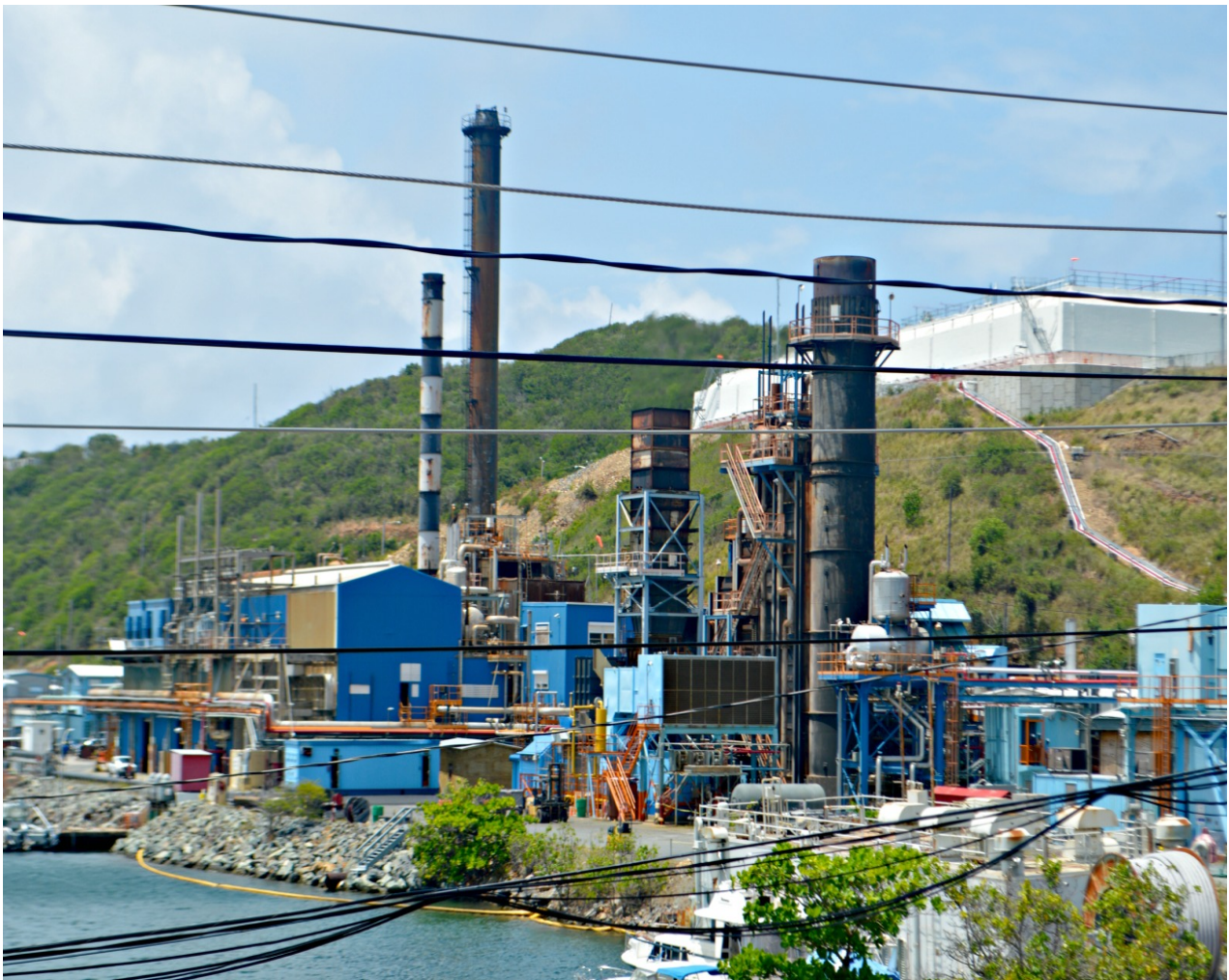
Randolph Harley Power Plant in St. Thomas By. ERNICE GILBERT FOR VI CONSORTIUM
