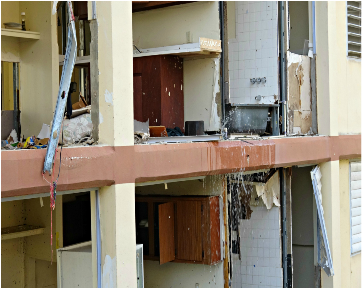
Tutu High Rise after Hurricane Irma's devastation on St. Thomas. By. ERNICE GILBERT FOR VI CONSORTIUM
