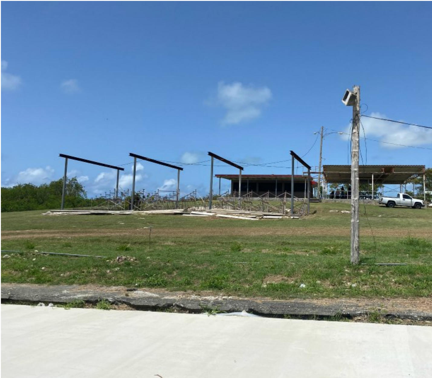
Hurricane-damaged drag racing bleachers and building on St. Croix. (Ernice Gilbert/VI Consortium)
