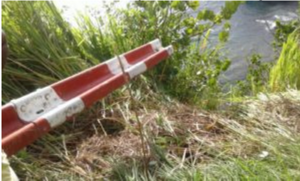
Broken railing that gave away during accident.
