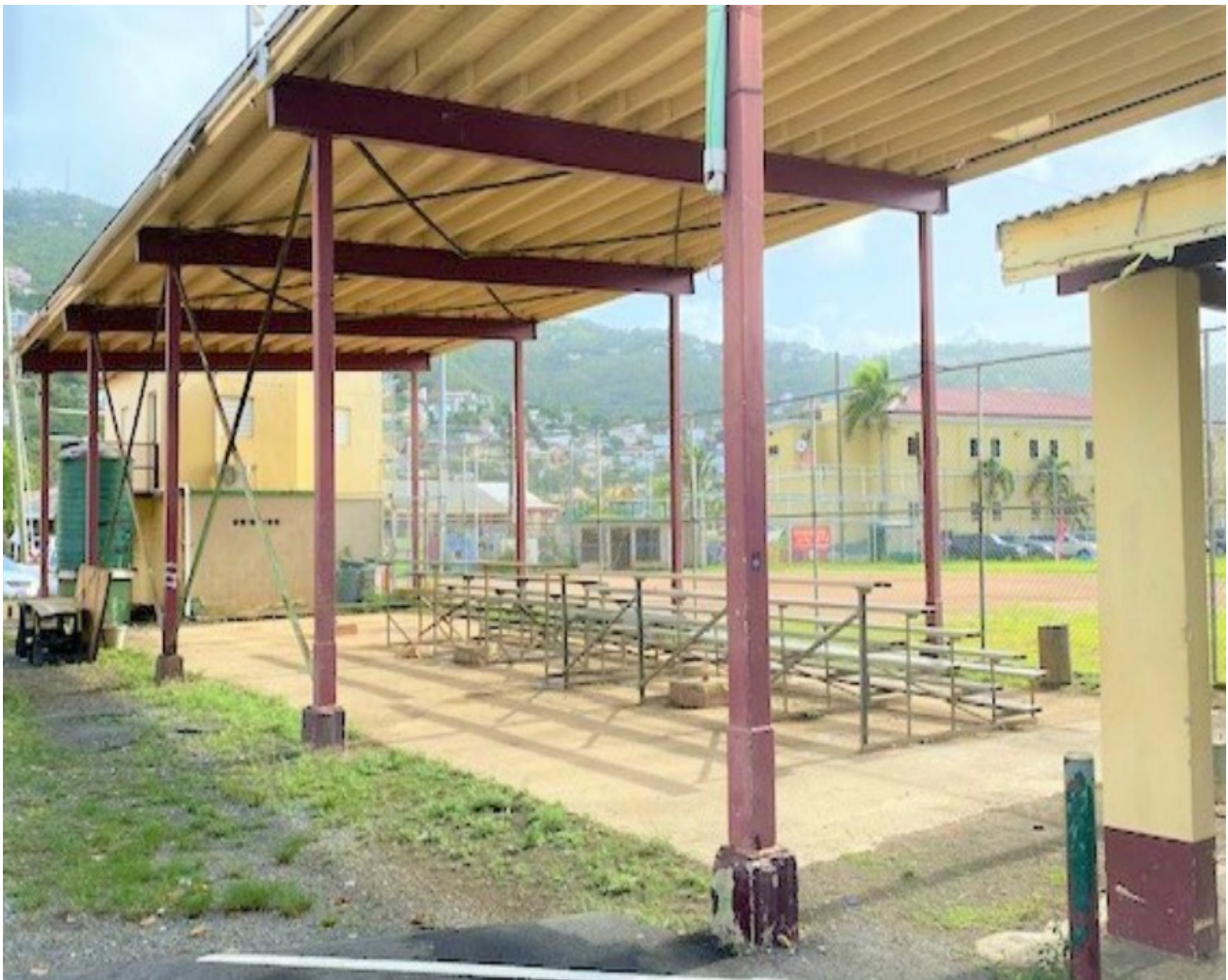
Aubain Ballpark Facility By. OFFICE OF DISASTER RECOVERY
