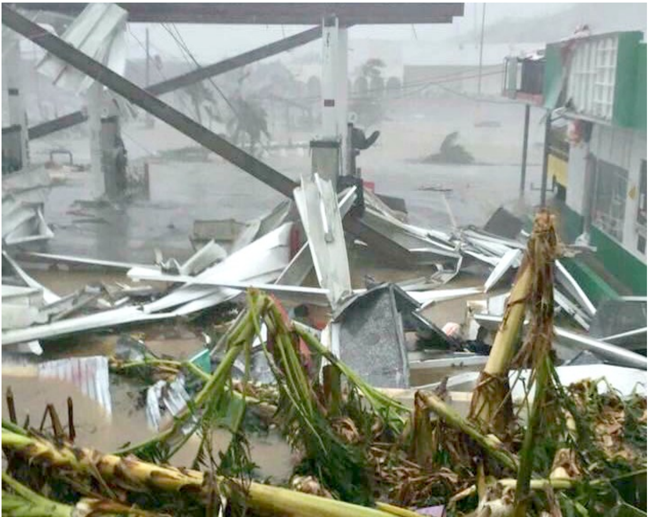
Hurricane Irma's Destruction in St. Thomas in 2017
