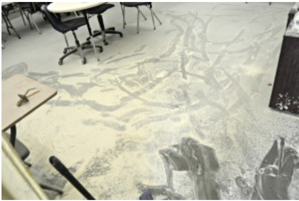
Floor of vandalized classroom, dirtied with fire
