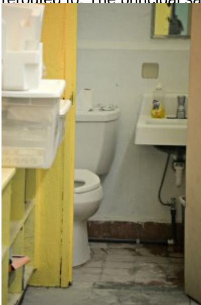
A vandalized restroom inside an affected classroom.
