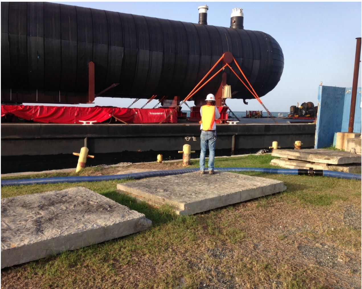
WAPA employee looks on as barge arrives at plant
