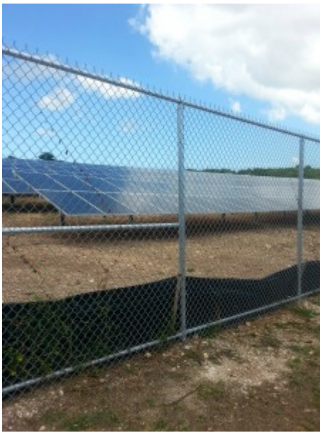
A portion of the 16,748 solar panels installed in Spanish
